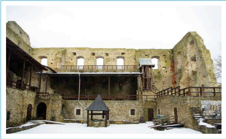
Image No. 3, Before the works. In 2014, the castle walls and later additions were in emergency condition. Photo SALM.
