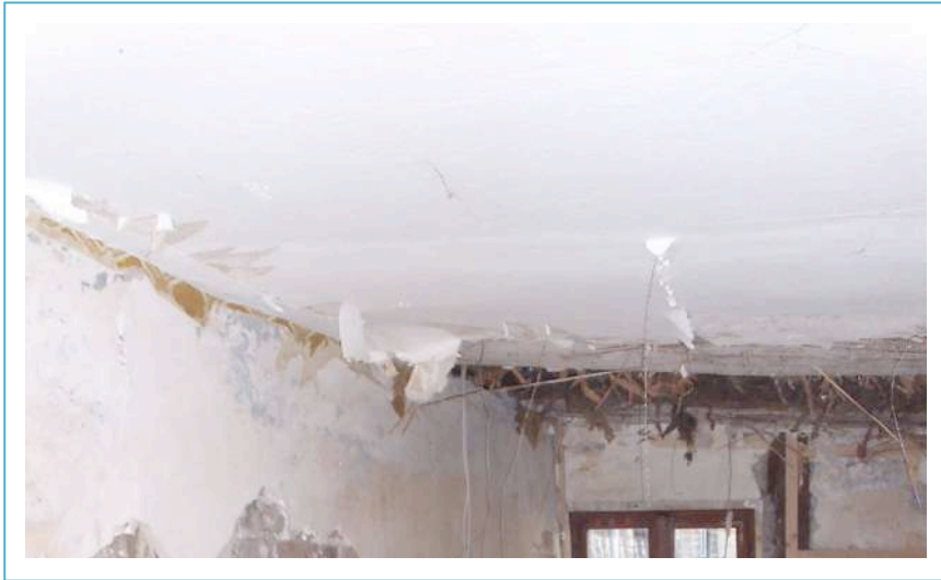
Image No. 3, upper floor with deformations and low room height, © LAKD M-V, LD, Jan Schirmer
