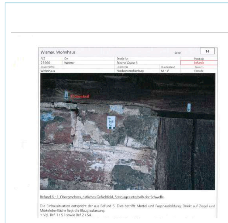
Image No. 11, 1. 1 st upper floor, eastern compartment field, stone layer below the sill, © Restoration examination, Lange, Wismar, 2015
