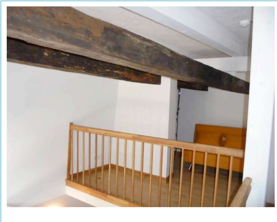
Image No. 19, mezzanine above the new gallery, © LAKD M-V, LD, Jan Schirmer
