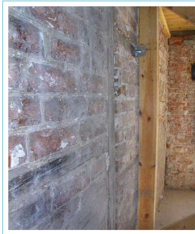
Image No. 16, the eastern gable wall with half-timbered construction, © LAKD M-V, LD, Jan Schirmer
