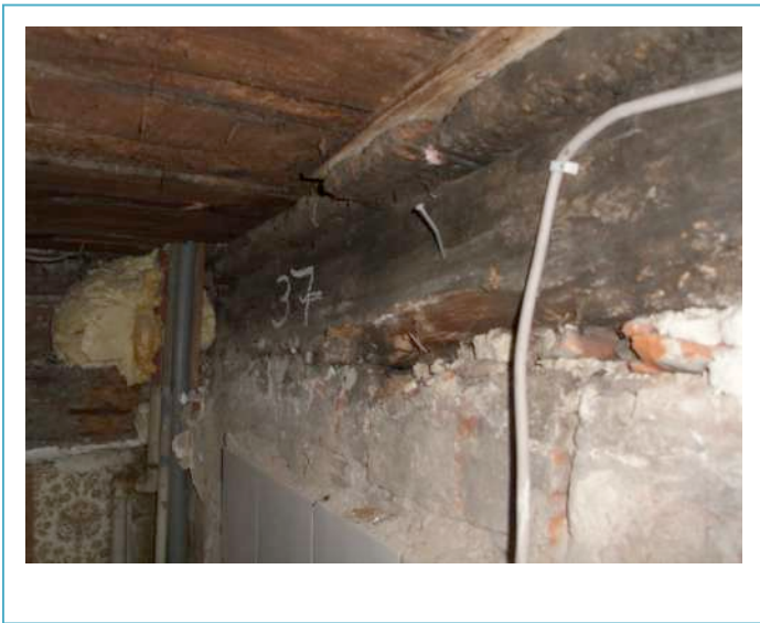
Image No. 17, the eastern gable wall with remains of the historical flooring of the adjacent building, © LAKD M-V, LD, Jan Schirmer
