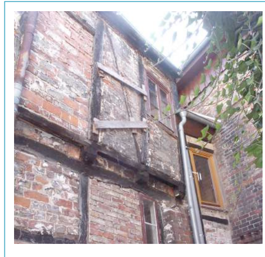
Image No. 5, courtyard facade, upper floor with traces of reconstruction and partly original infill, original supporting post © LAKD M-V, LD, Jan Schirmer
