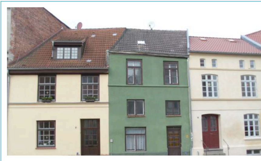
Image No. 1, Frische Grube 5 with green facade colour before restoration 2013, © LAKD M-V, LD, Jan Schirmer
