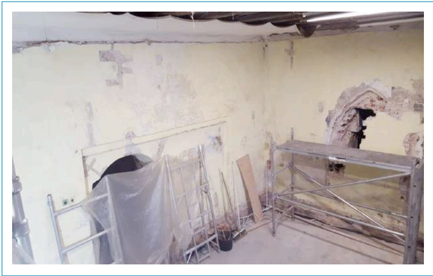
Image No. 4, The west and north walls of the sacristy before the conservation work.
