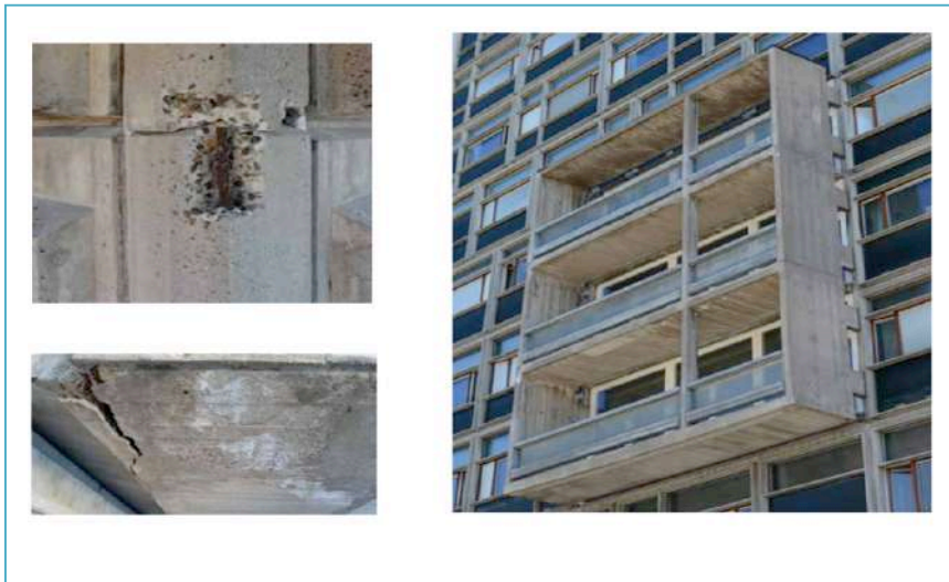
Injuries on the concrete elements and on the balconies in concrete. Photo: Sven Olof Ahlberg.
